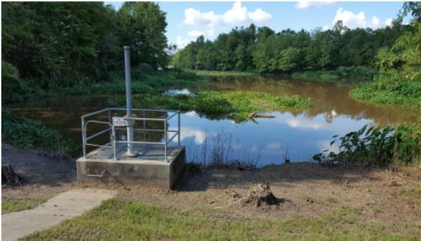
Existing 54" Gate at Bayou Courtableau That Provides Freshwater to Bayou Ami-Borrow Pit
