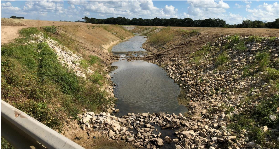
Ile Des Cannes after to Channel Improvements (South of Old Spanish Trail)
